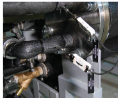
Temperature sensors for the PD cylinder and Temperature Control System
